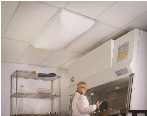
Fabric Air Distribution In Laboratory (“LabSox” Photo Courtesy of DuctSox Corporation)
