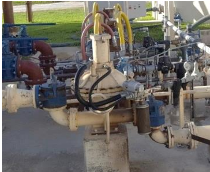
Figure 16: Air diaphragm pumps with compressed air hoses in black, red, and yellow.
