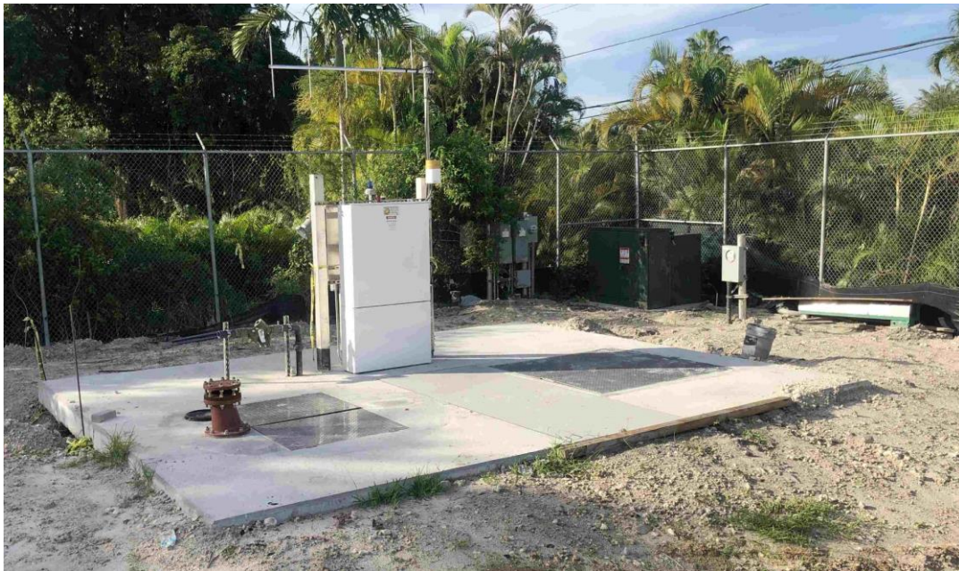
Figure 9: Top, wood forms for a concrete slab to surround the wet well (left) and valve vault (right). Final installation with vent (red), control panel, and communications antennae.
