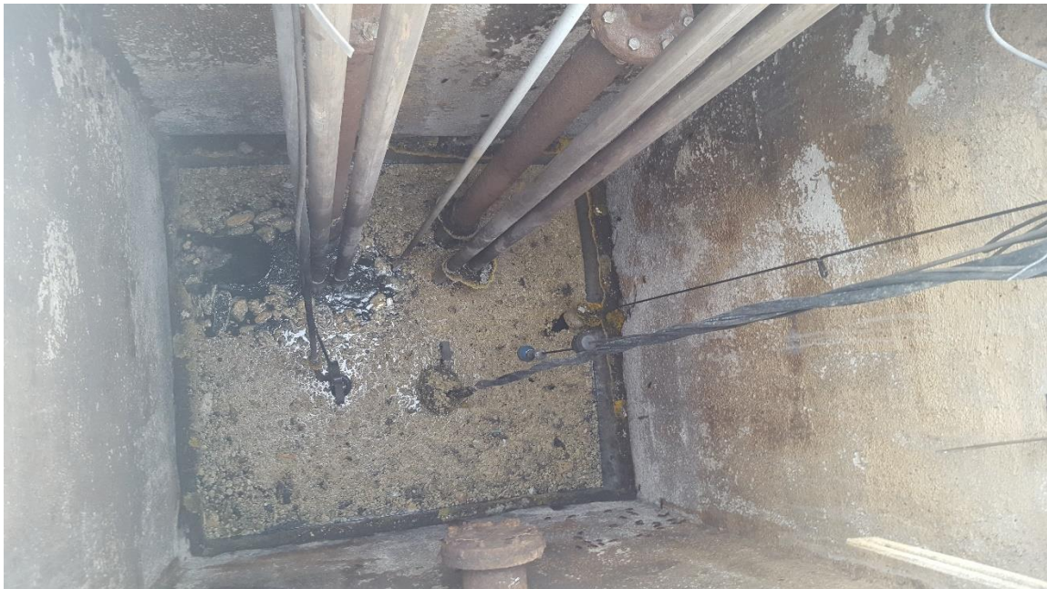
Figure 8: Looking down inside a rectangular wet well with two pumps on slide rails. The tops of the two pump motors are visible in the wastewater. Floats are hanging from a cable rack on the right.
