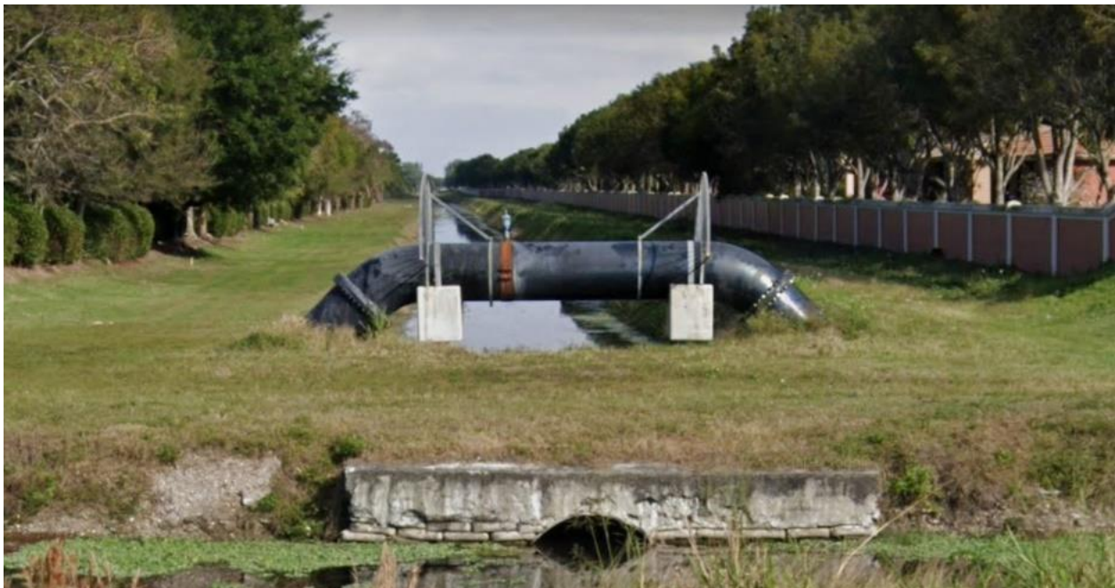
Figure 2: A force main crossing over a canal with an air relief valve in blue.
