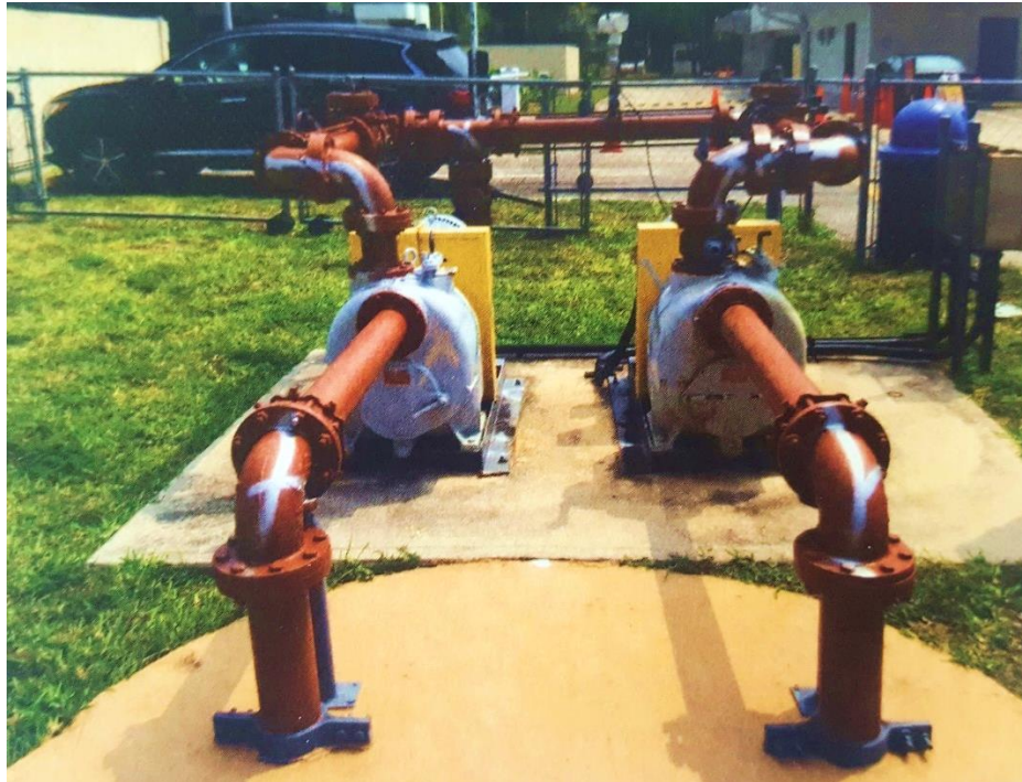
Figure 15: A suction lift station with self-priming pumps mounted on an outdoor slab.
