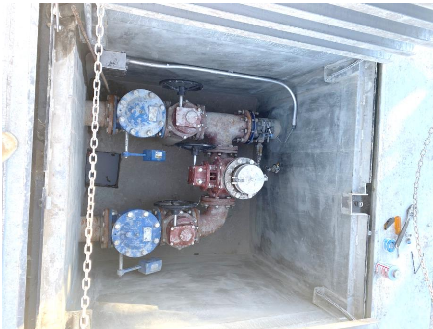
Figure 7: A valve vault with two check valves (blue), plug valves (red), a pump-out connection on a riser, and a pressure gauge on the force main (to right).
