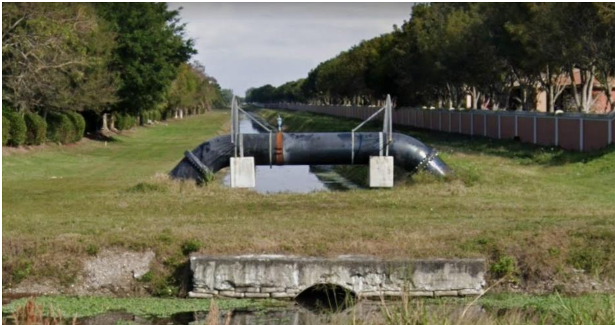
Figure 2: A force main crossing over a canal with an air relief valve in blue.
