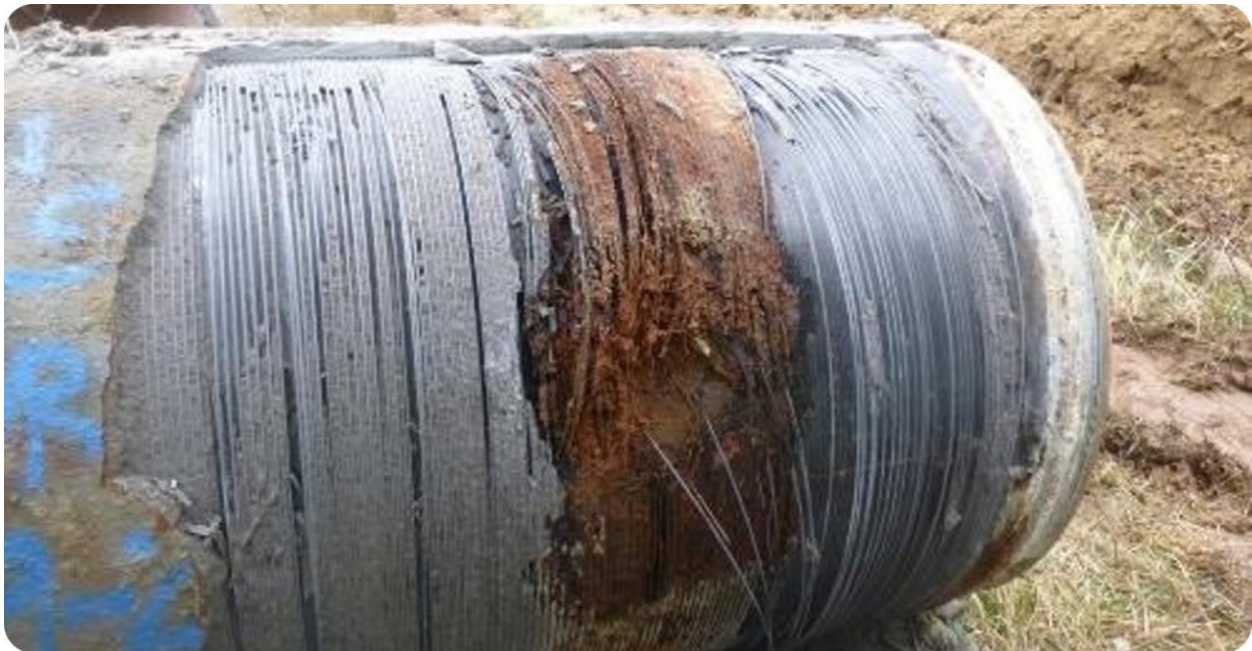
Figure 19: A section of prestressed concrete cylinder pipe (PCCP) with wire damage discovered by internal electromagnetic scanning.
