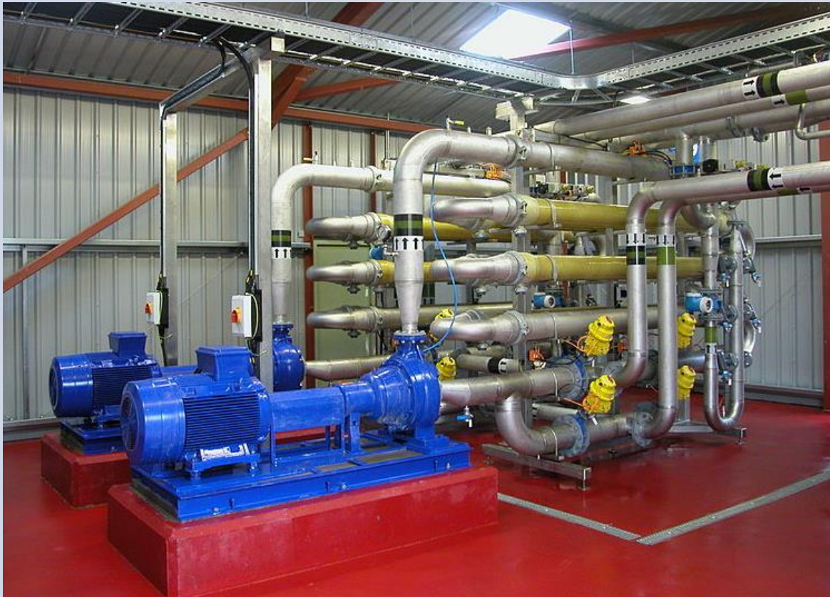
Figure 12: Two skids with ultrafiltration membranes (green tubes) and high-pressure feed pumps (blue).
