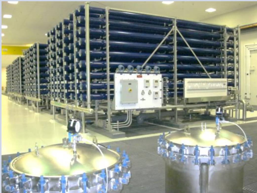
Figure 13: Large water plant with four RO skids, each with (81) blue RO tubes. Two upstream cartridge filters are seen in the bottom.
