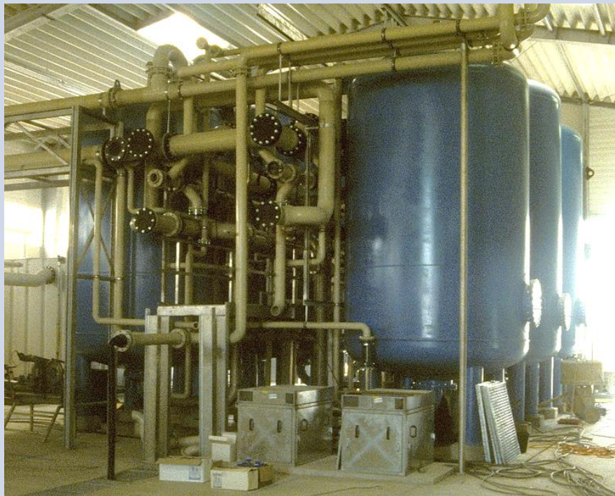
Figure 9: Activated carbon adsorption system for water treatment, with six vessels. Each vessel can be isolated to replace the media inside.
