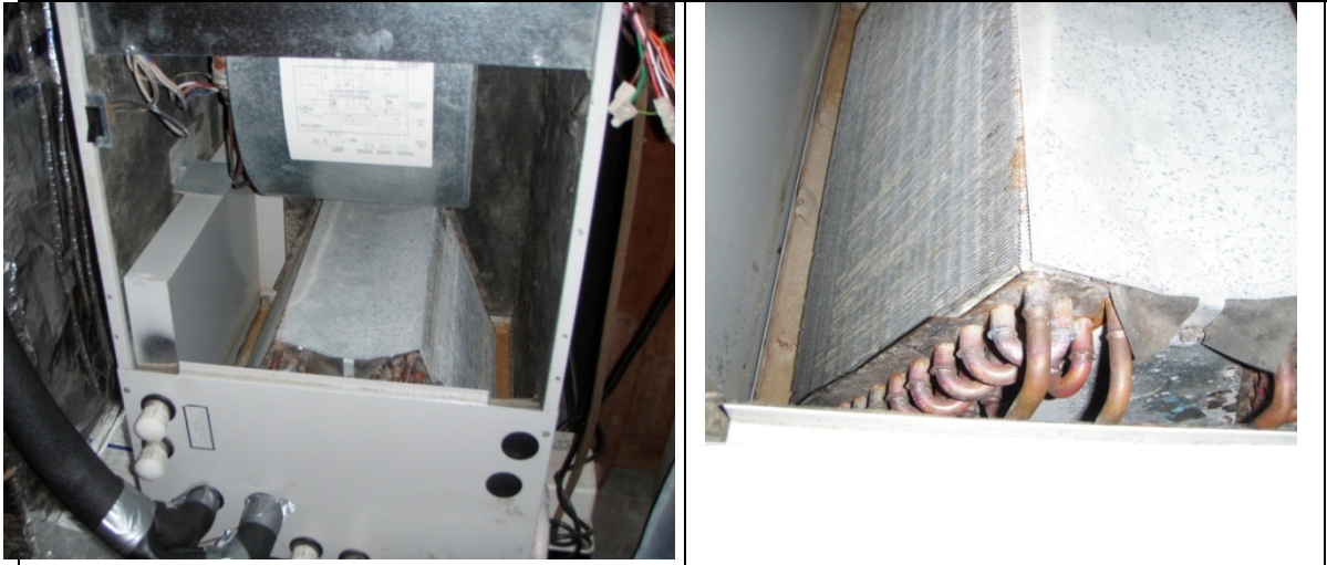
Condenser detail within the air handler cabinet.
