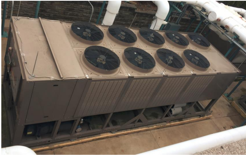
Figure F-14 (A Picture of an Air Cooled Chiller)
