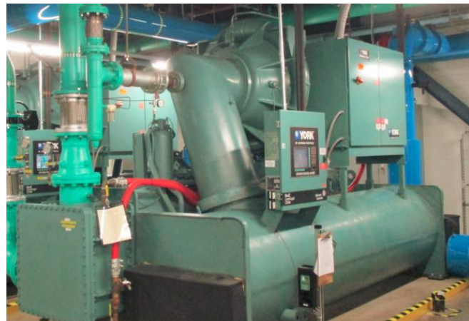
Figure F-15 (Pictures of a Water Cooled Chiller)
