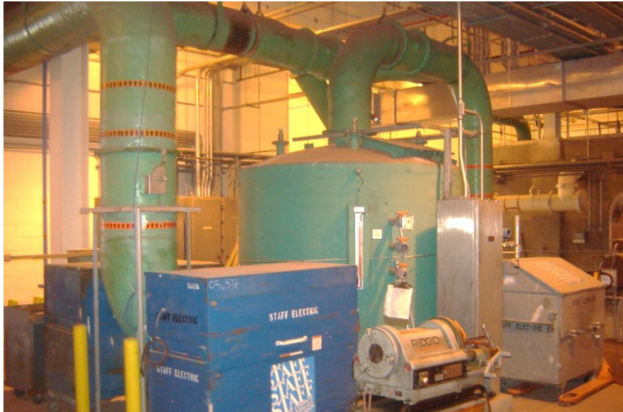
Figure 19: Odor control vessel (green, center) with a manometer (white with red stripe) and three sample ports with PVC valves.
