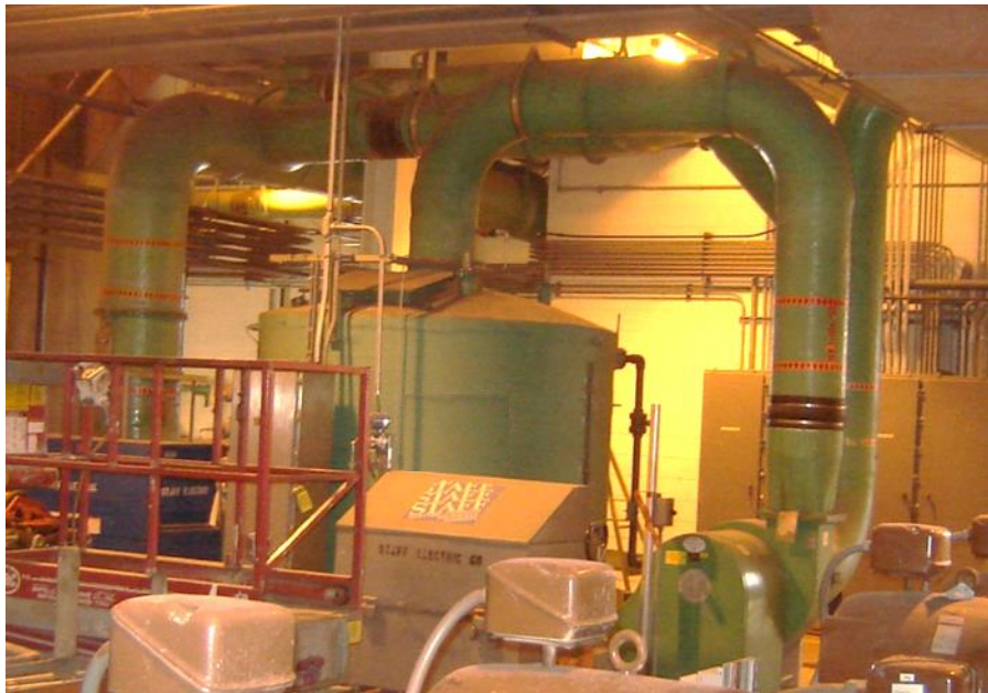
Figure 18: Odor control enclosure (green, center) and air fan (green, right).
