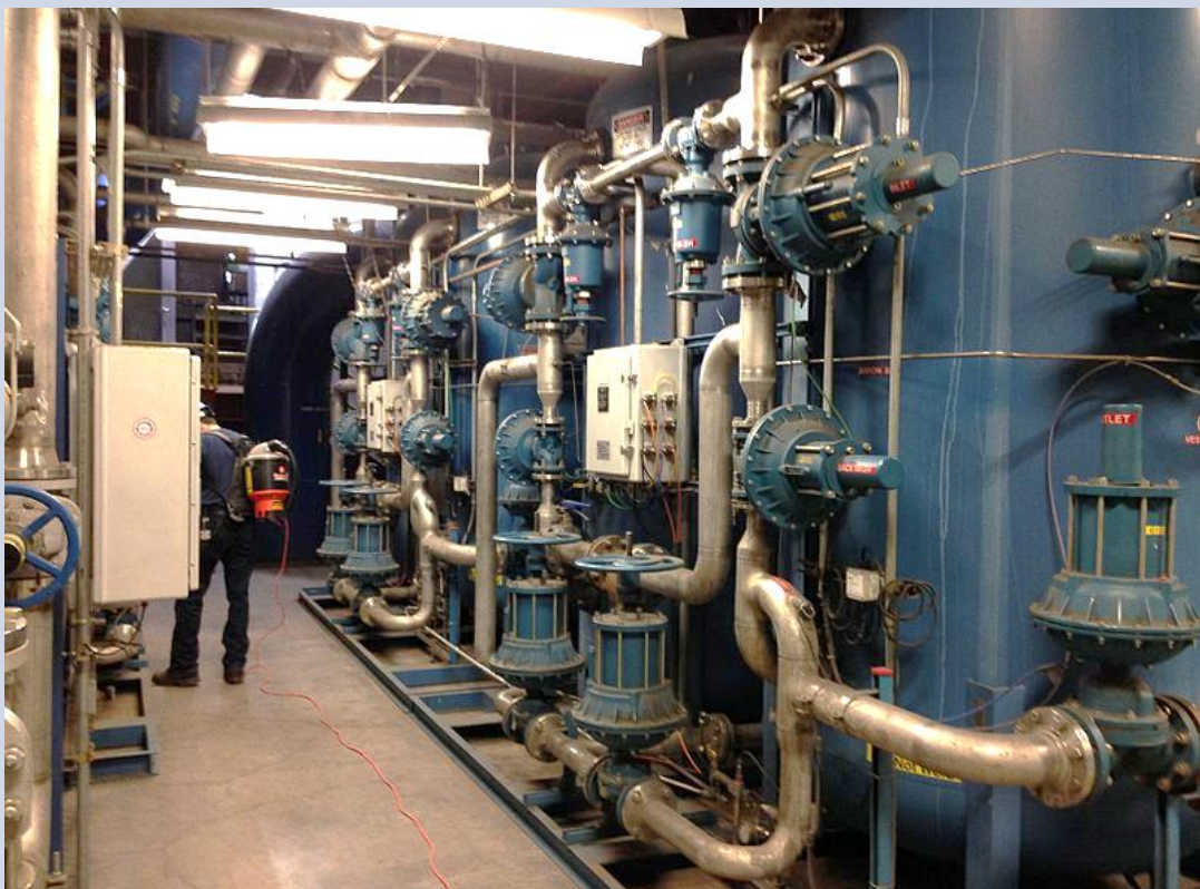
Figure 8: Four fixed-bed ion exchange vessels in blue with piping and valves to allow for treatment and backwash cycles.
