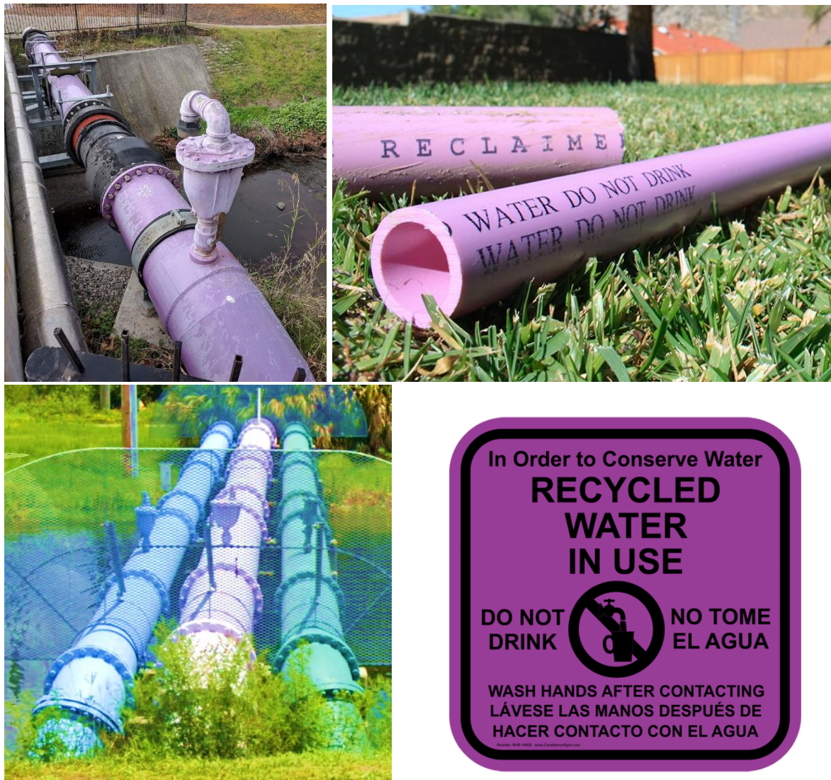
Figure 13: Upper left: A purple pipe in Mountain View, CA. Upper right: Reclaimed pipes with labels. Lower left: Portable main (blue), reclaim main (lavender), & force main (green).
