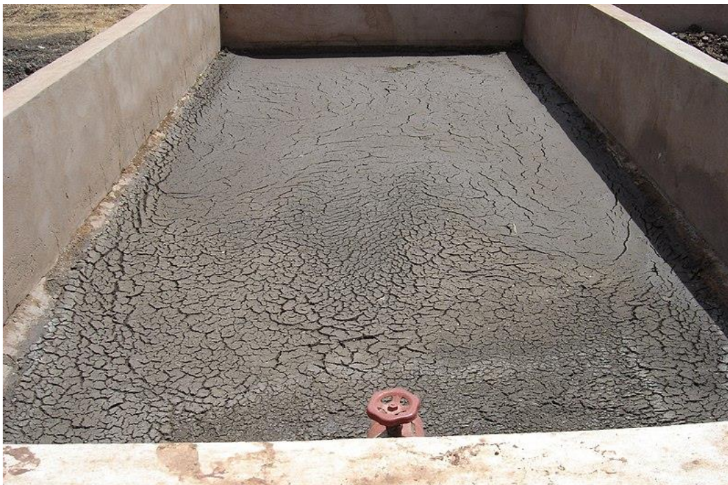
Figure 8: Sludge being dried by evaporation in a sludge drying bed.
