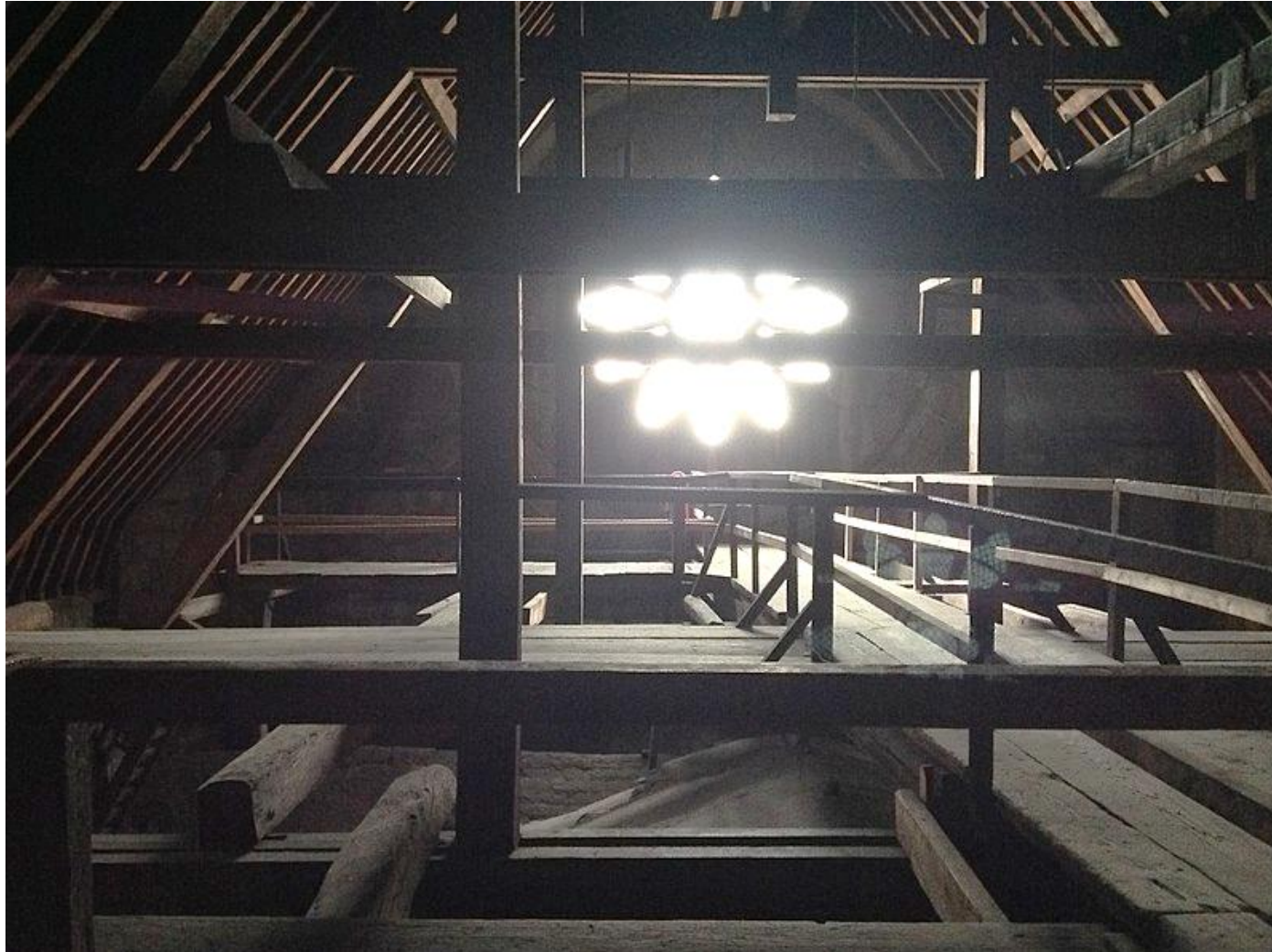
Figure 4: Attic of the Notre-Dame Cathedral with wooden frames and no fire sprinkler system.
